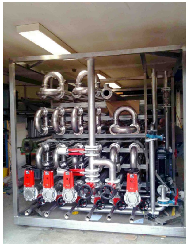
Almost finished system in workshop.
